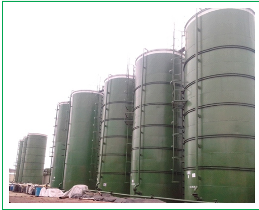
VERTICAL MUD TANKS
